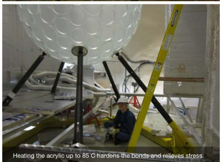
The oven was assembled around the AV a total of five times.
