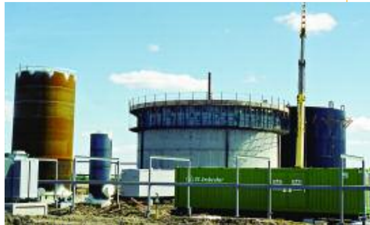
The IMUS project in Vegreville, Alberta.
