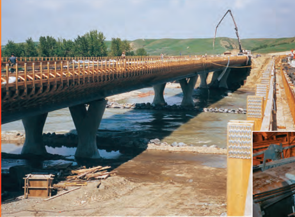
Top left : Construction of Bow River bridge for Deerfoot Trail extension south of Calgary
