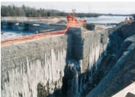
Excavation for a low head hydro project on the Trent Severn Canal near Batawa, Ontario.
