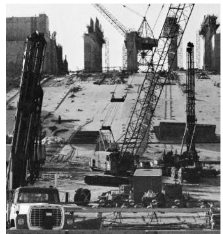
Installing anchors on the spillway of a major dam on the Saskatchewan River.
