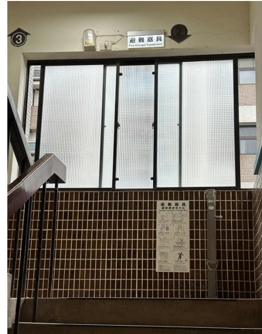
Fire Escape Equipment
