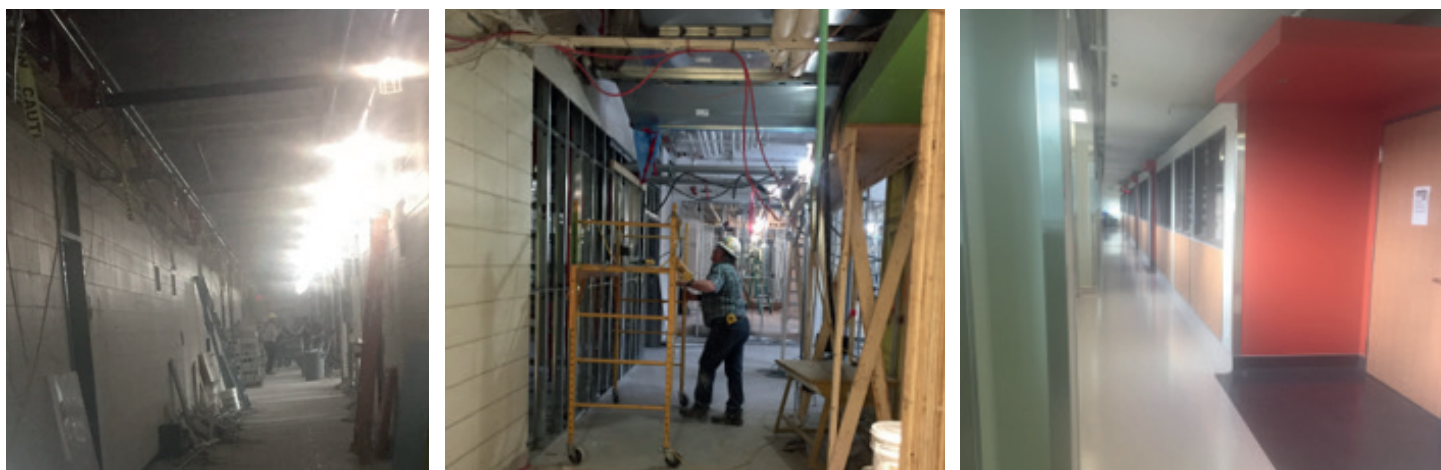
Demolition (left), renovations of Chem West South in progress (centre), and the new look coming in 2018, based on Chem West North (right).
