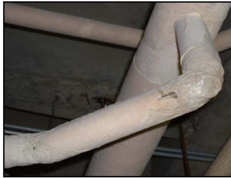
Pipe elbow mud wrapped with non-painted
