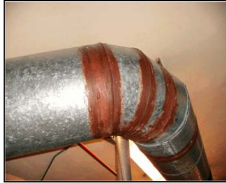
Red duct mastic
