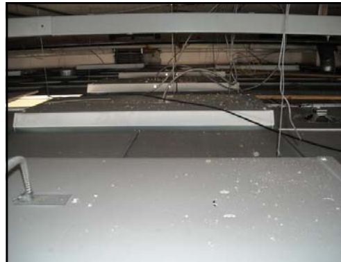
Texture coat debris on ceiling tiles & light fixtures
