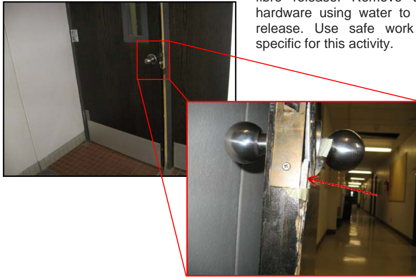
Fire door interior (white sheets of asbestos)
