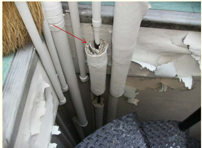
Corrugated "Aircell" pipe run insulation – Dentistry Pharmacy Centre
