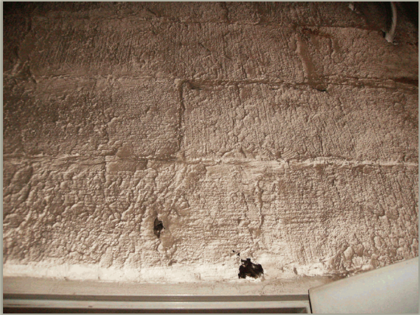
Mastic/cork mixture on a block wall – Chemistry Centre West
