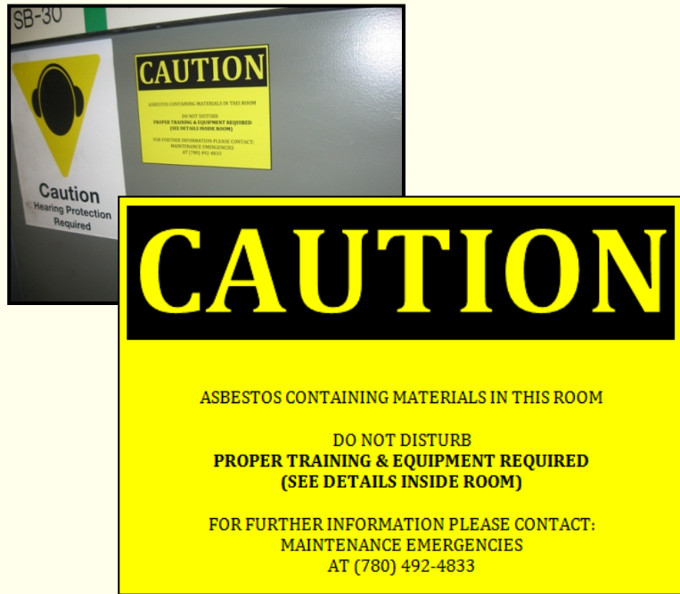
Label posted on door to mechanical room containing asbestos materials
