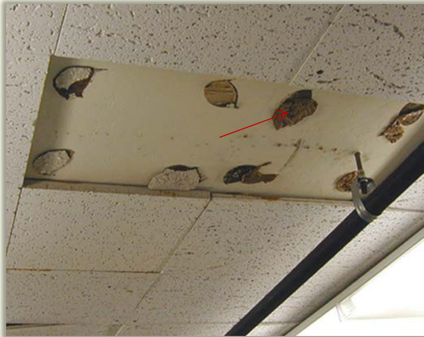
Ceiling tile mastic – Biological Sciences Building
