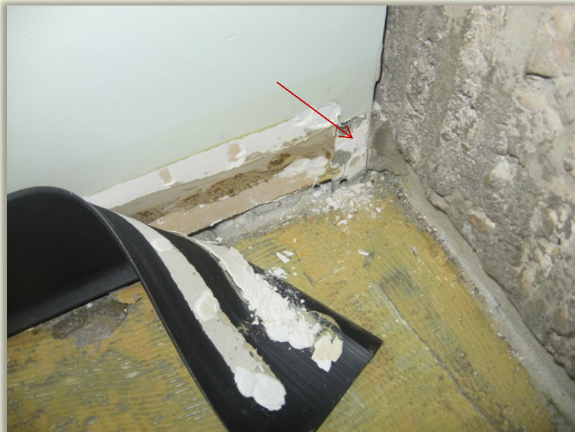
Drywall joint compound – Law Centre
