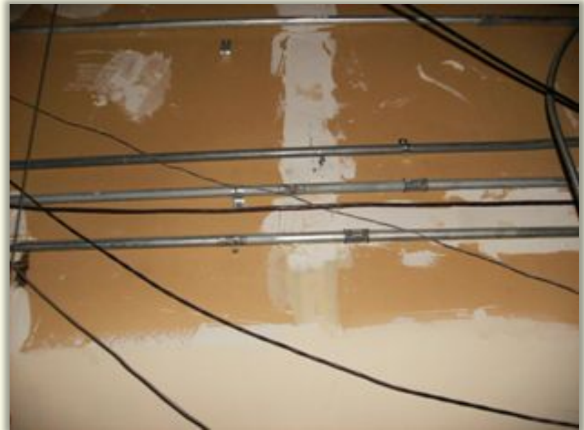
Drywall joint compound – General Services Building
