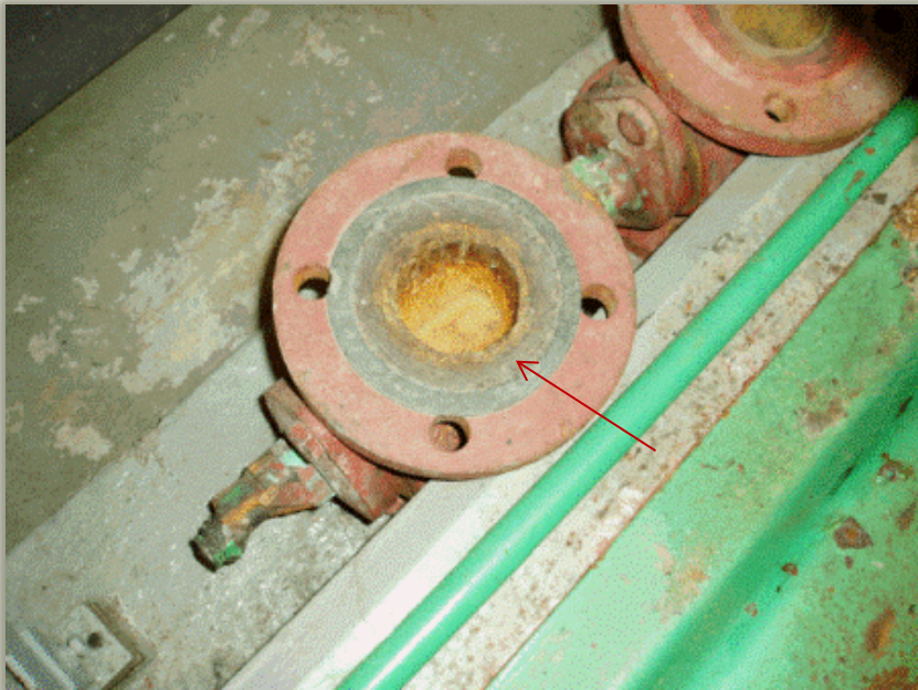
Gasket – H.M. Tory Building
