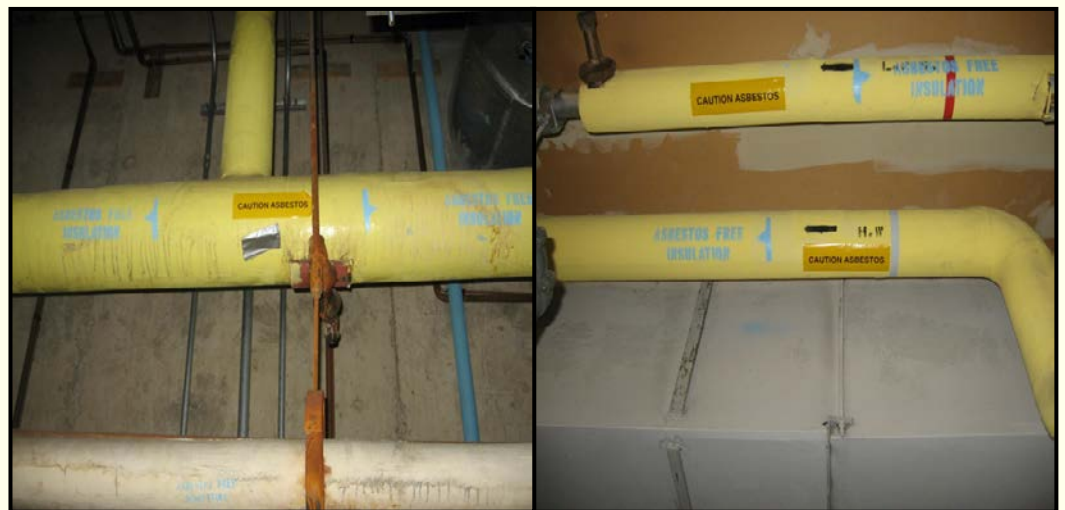
Labels and stencils indicating transition from asbestos to non-asbestos insulation
