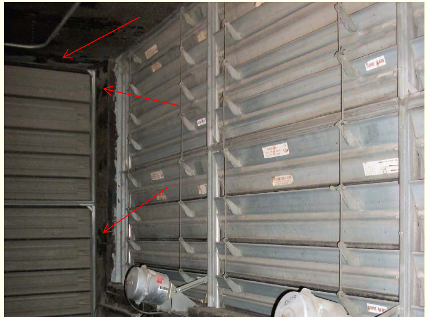
Mastic on fiberglass sheets inside Air Handling Unit – Athabasca Hall
