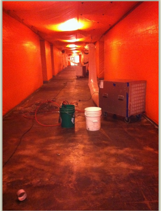
Inside a high-risk containment for the abatement of asbestos containing floor tile and floor levelling compound
