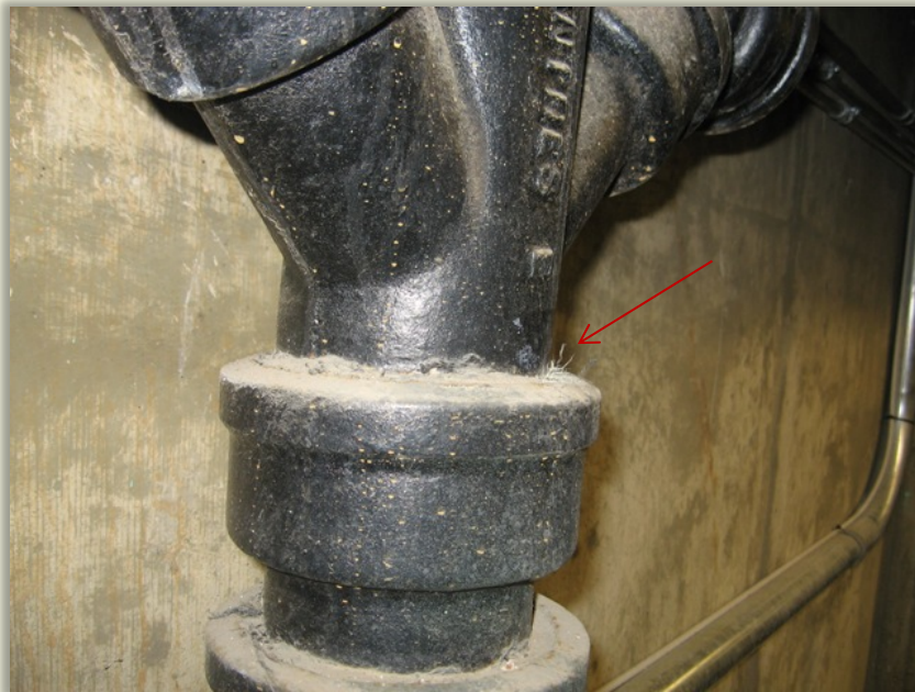
Joint packing on a cast iron pipe – Chemistry Centre West
