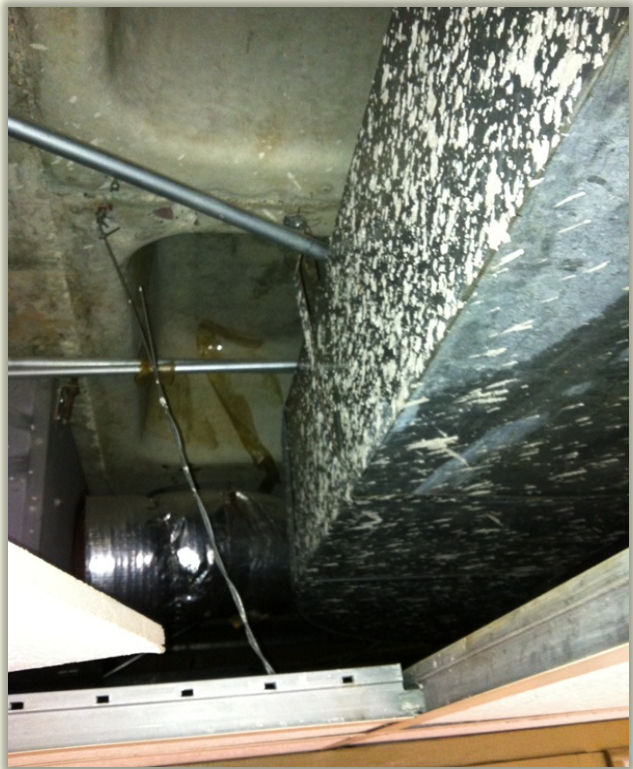
Ceiling texture overspray on duct and concrete structure – Education Centre - North
