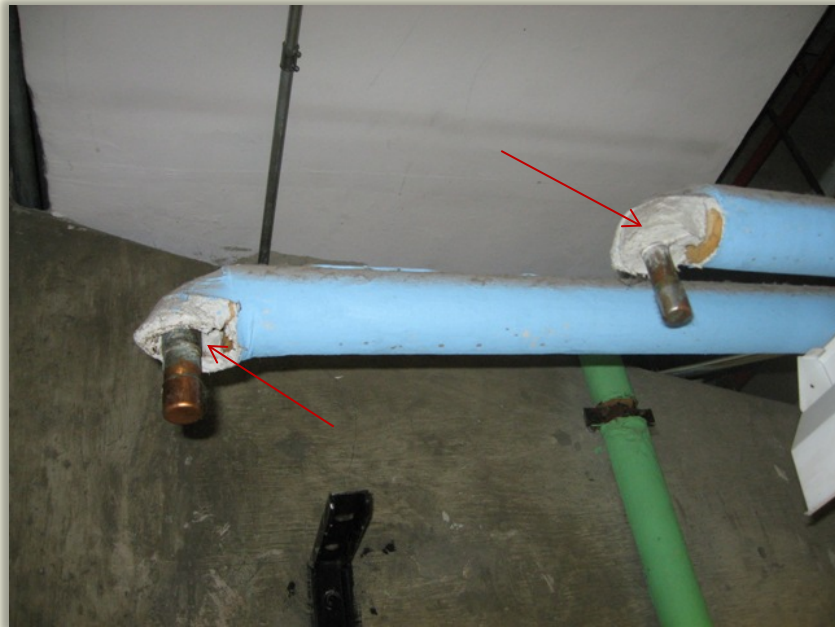
Pipe fitting insulation – H.M. Tory Building
