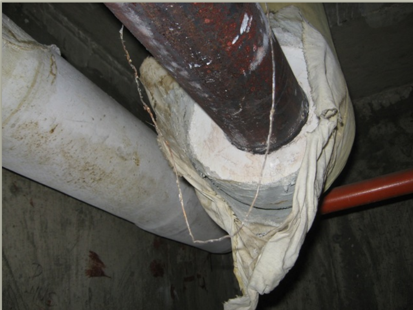
Block pipe run insulation – H.M. Tory Building
