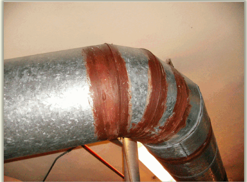
Mastic on ductwork – Chemistry Centre West
