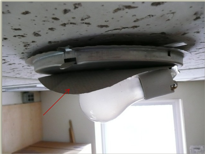
Paper insulation on incandescent light fixture – Pavillon McMahon (Campus Saint-Jean) (abated)
