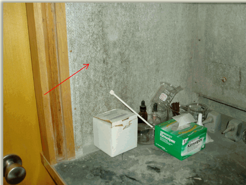
Cement board (transite) inside a fume hood – H.M. Tory Building
