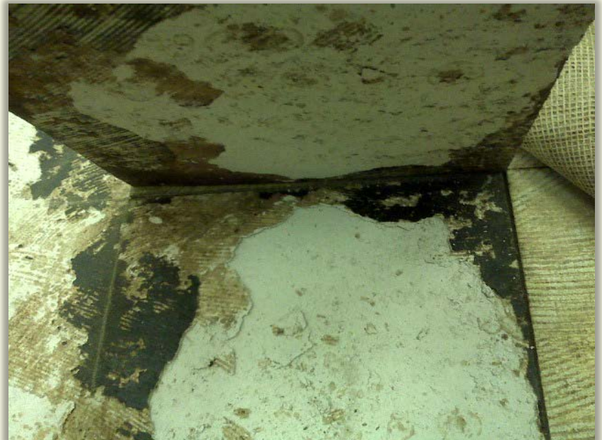
Cement-like floor levelling compound – Education Centre North
