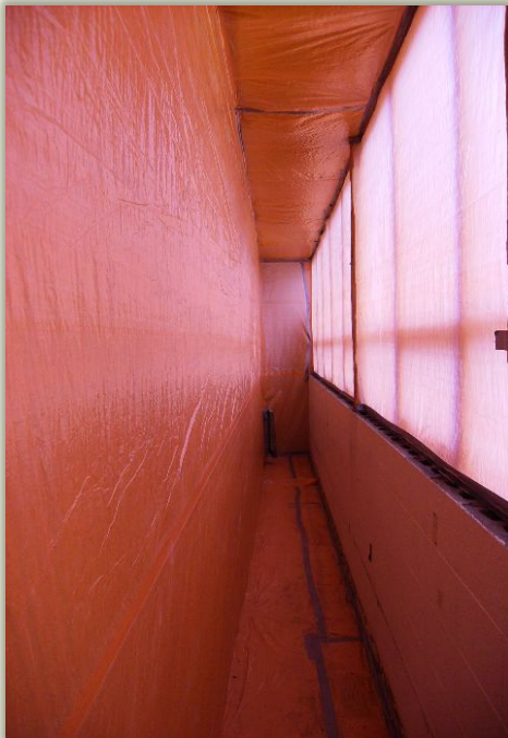
Inside a high-risk containment for the abatement of asbestos contaminated vermiculite from a block wall
