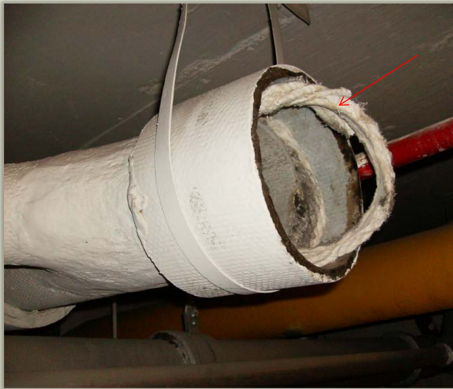
Joint packing around transite duct joint – Chemistry Centre - West
