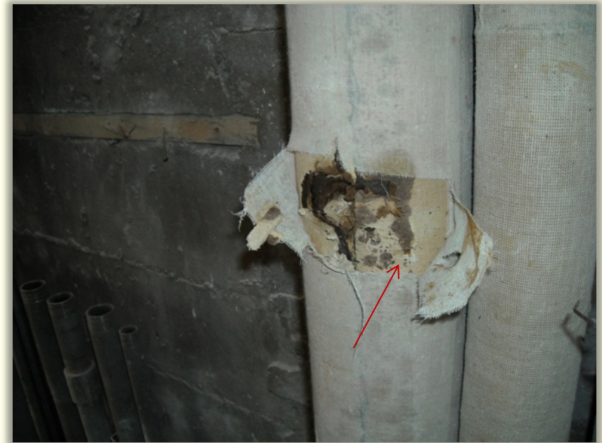
Construction paper pipe insulation – University Hall
