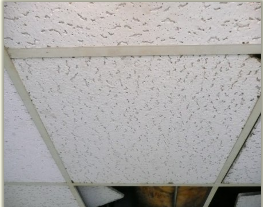
2'x2' T-bar ceiling tile – Pavillon McMahon (Campus Saint-Jean)
