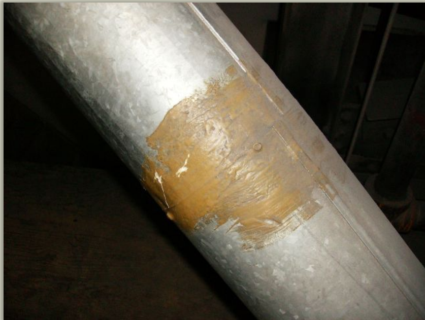
Mastic on ductwork – North Power Plant
