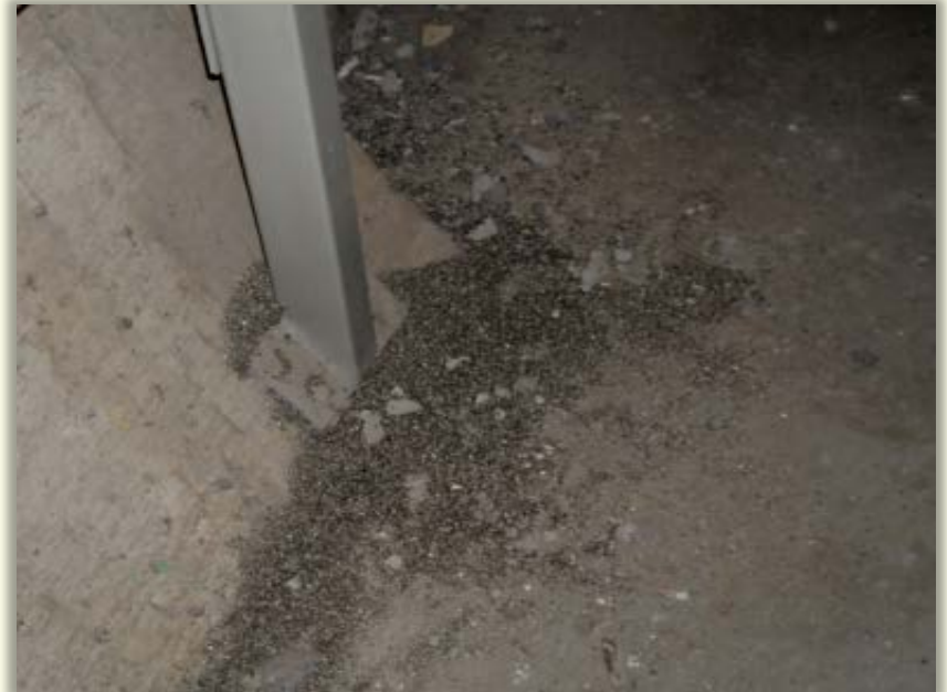
Loose black vermiculite from block wall cavity – RCMS Building
