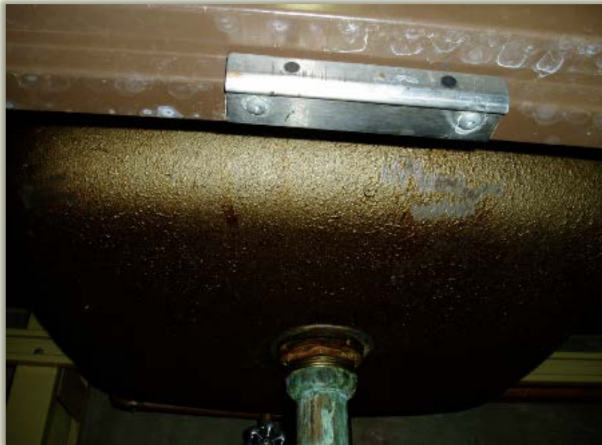
Mastic on sink basin – Mechanical Engineering Building
