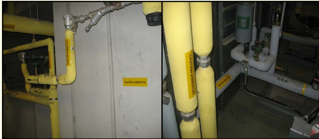
Labels applied to asbestos containing pipe and duct insulation
