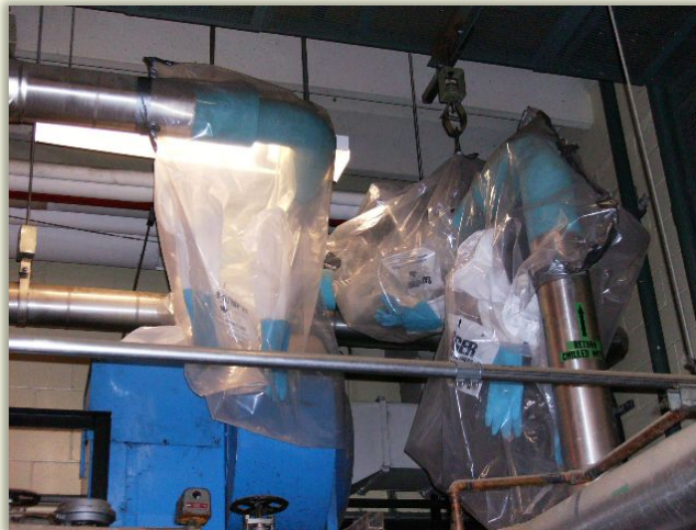
Glovebags used to perform localized abatement of asbestos containing pipe fitting insulation
