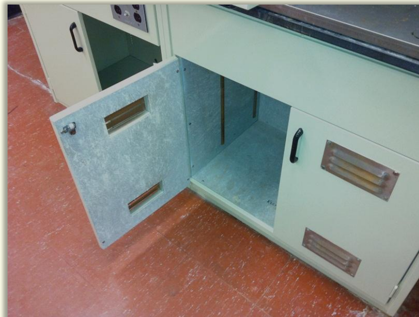
Cement board (transite) inside an acid cabinet – Chemistry Centre - East
