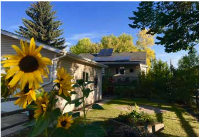
Ardelle Ries and Roger Admiral’s newly installed solar panels. Photo courtesy of Raj Rathnavalu.
